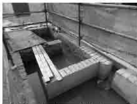
项目区汇水口处三级沉沙池 (2016.9)
