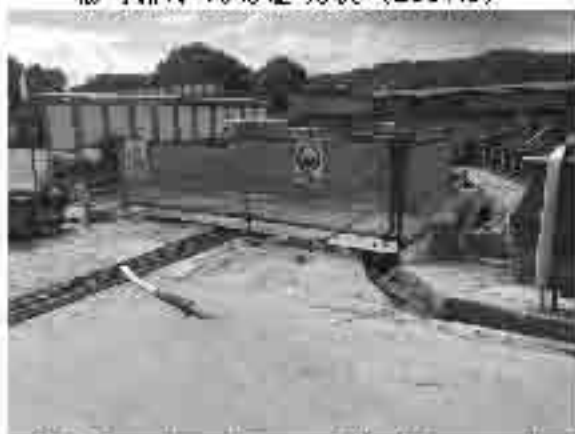
项目区汇水口处三级沉沙池 (2017.6)
